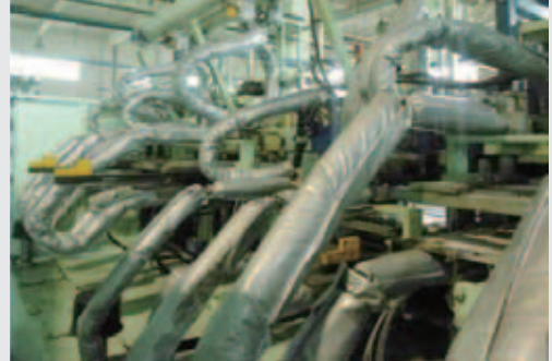
Insulation of factory machines resulted in significant energy savings
