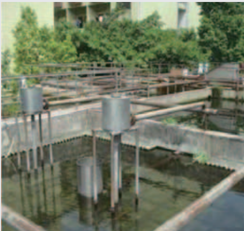
Water treatment system
