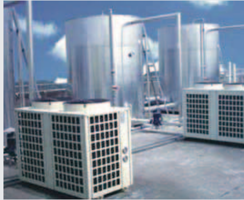
Reusing heat from machinery to power dormitories
