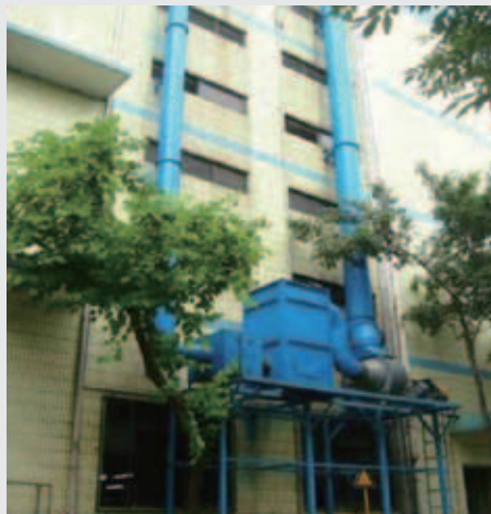
Carbon absorption device installed at one of our factories
