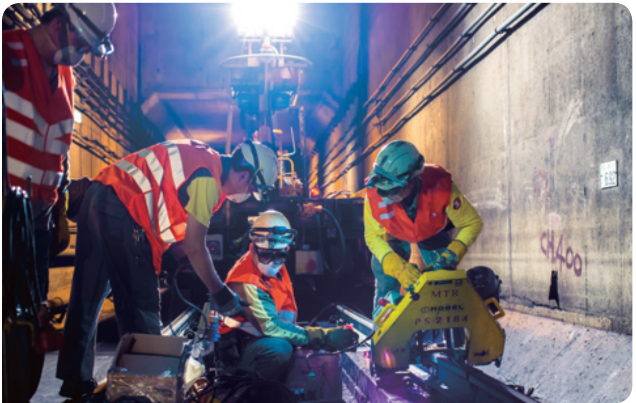
Extensive maintenance programmes ensure continued efficiency and reliability
