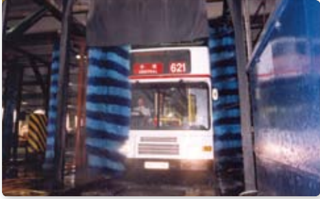
Our bus-washing machines were equipped with water recycling systems
