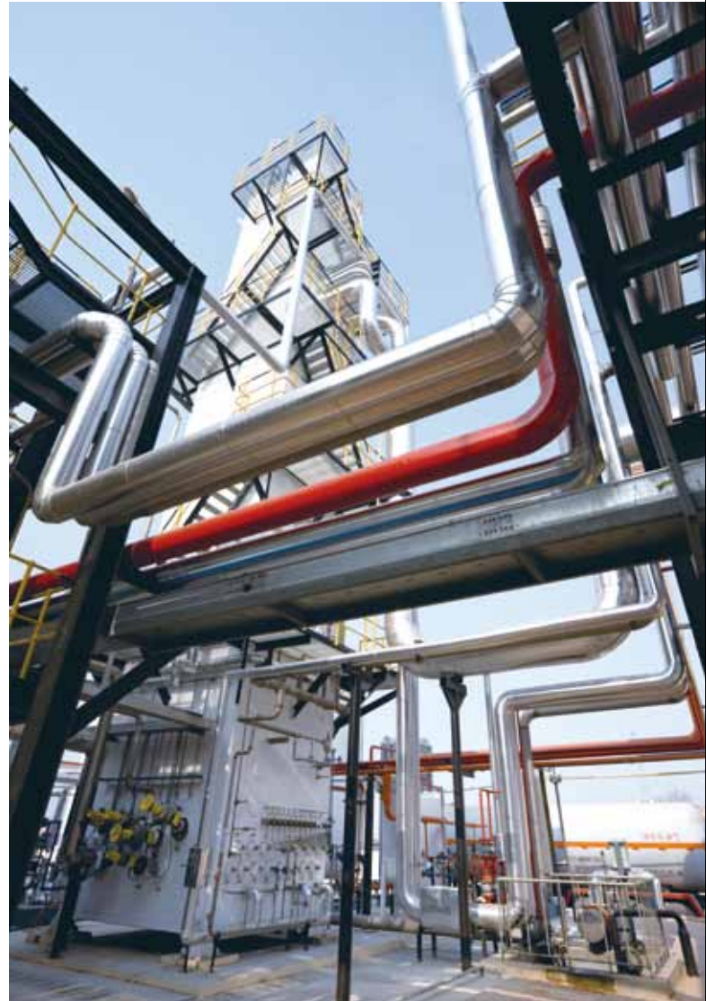
Liquefied coalbed methane (LCBM) plant in Shanxi province
