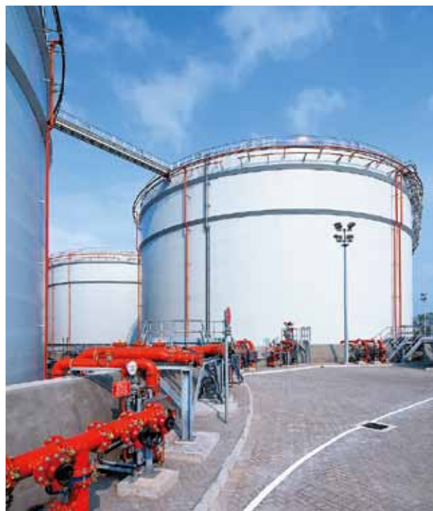
ECO Aviation Fuel Facility
