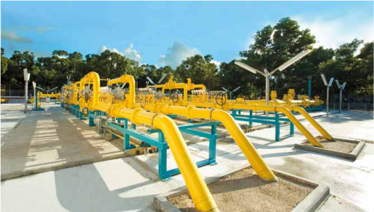
High-pressure submarine pipelines deliver natural gas from Guangdong to the Tai Po Plant
