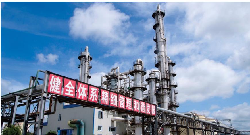
© Distillation towers of COFCO Bio-Energy (Zhaodong) Co., Ltd.
