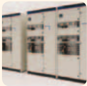
Building Automation and Security
