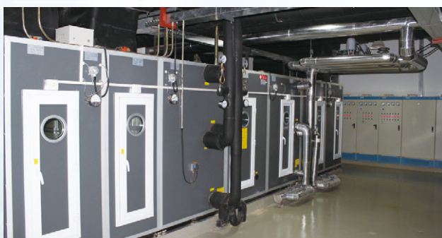
Air-conditioning purification system
