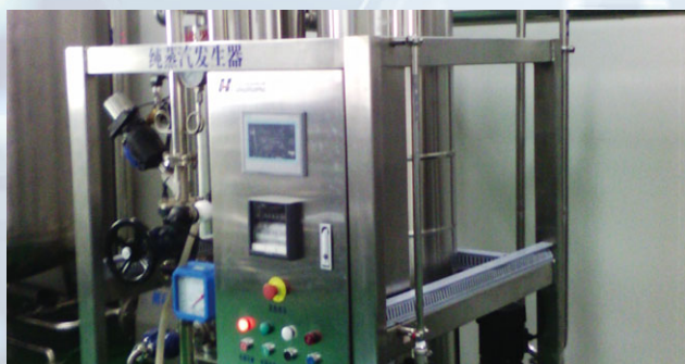
Equipment Name: Purified Stream Generator Description: Provide Purified Stream to Various Equipments
