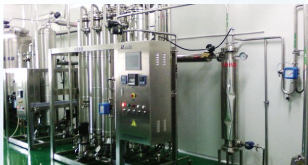
Equipment Name: Injection Water System Description: Provide Injection Grade Water
