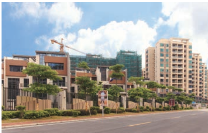
Partial view of town houses and apartments under Phase I of Metropolitan Oasis
