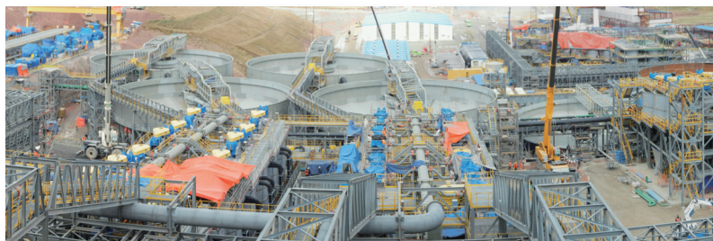
Flotation & Thickener Area
