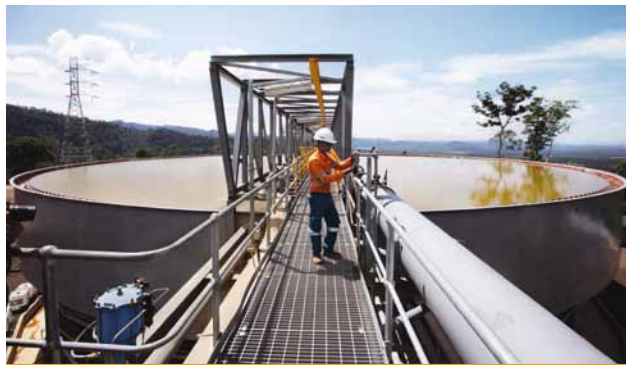
Employee monitoring the Water Polishing Plant process.
