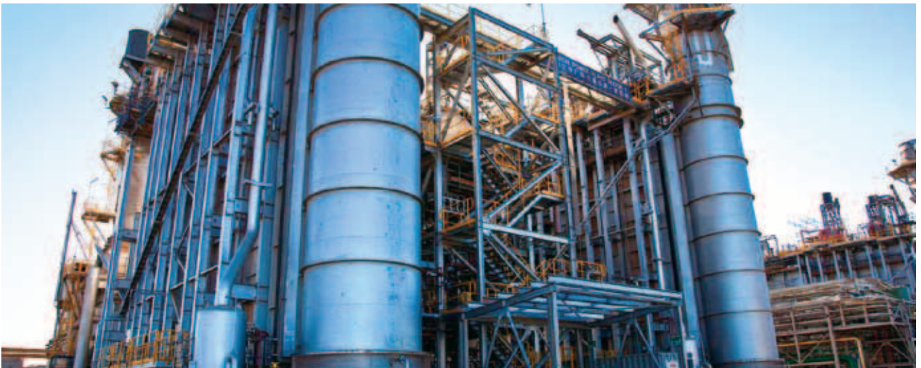
CPM – Combined-cycle Gas Turbine Power Station
