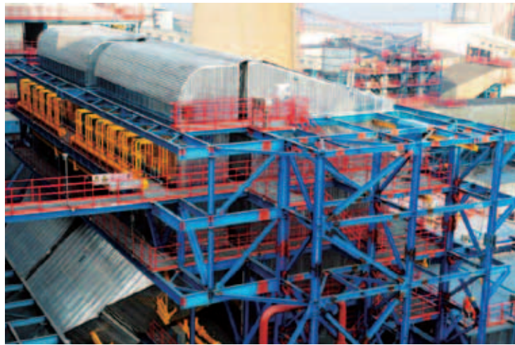
De-sulphuring System in Power Plants
