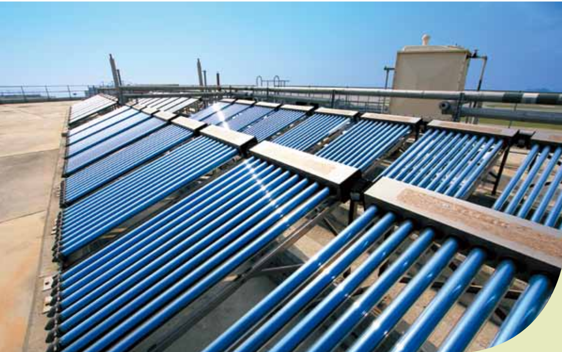
Solar water heaters installed on the roof of a hangar in HAECO
