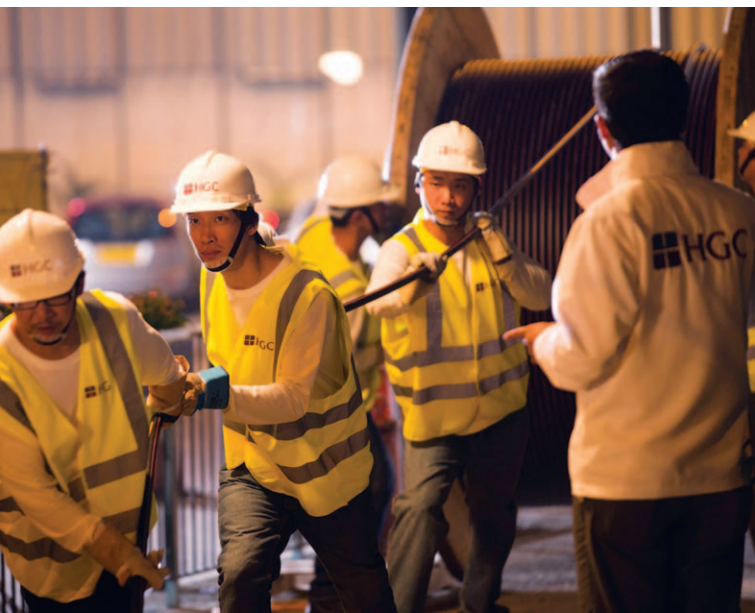
▶ Comprehensive network and connectivity services continue to serve HGC's broad customer base.
