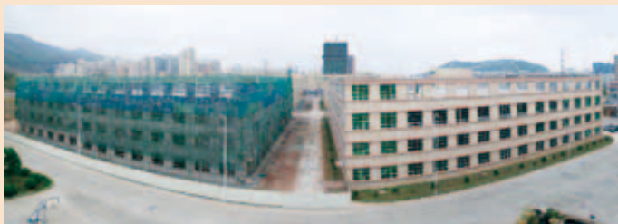
Daya Bay Industrial Complex under construction: Block 5 & 6 (operation has partially commenced) and Block 7 & 8 正在興建中的大亞灣工業園：第5、6棟(局部已經開始營運)及第7、8棟廠房
