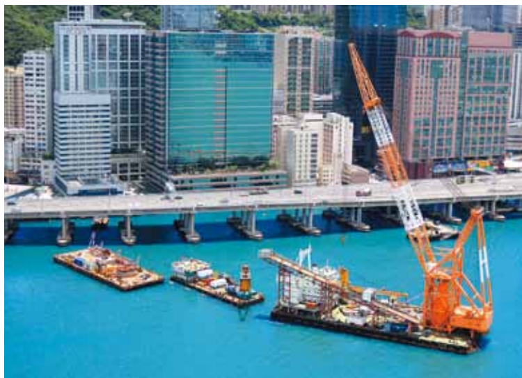
To cope with the Government's development of South East Kowloon, we relocated a twin submarine pipeline between To Kwa Wan and North Point.
