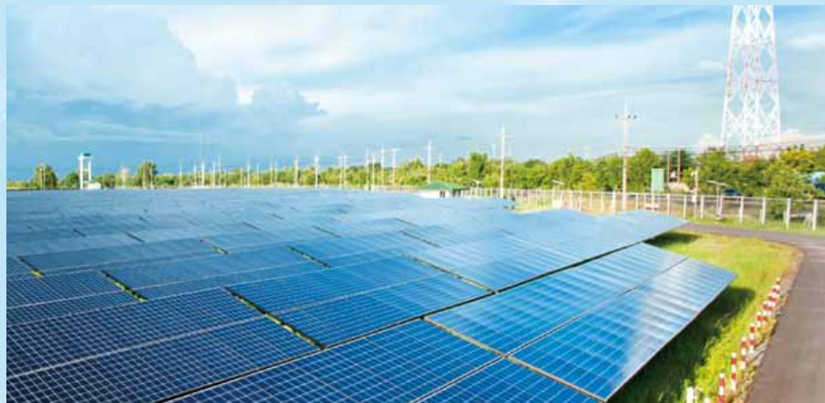
A glance of the photovoltaic site 光伏現場實景一瞥
