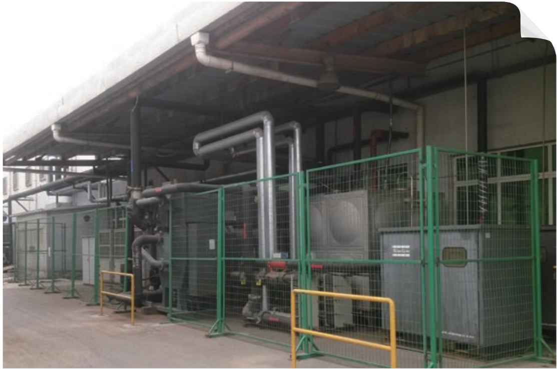
The waste heat utilization equipment in Tianjin company
