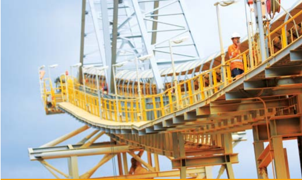
Crushed ore feed conveyor to the process plant.
