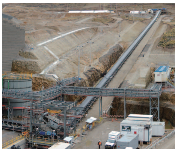
Conveyor No.1 & No.2 and Transfer No.01
