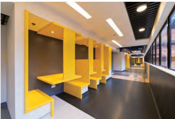
Spatial reorganisation works to Core FJ, 7/F of The Hong Kong Polytechnic University 香港理工大學七樓Core FJ的重組工程
