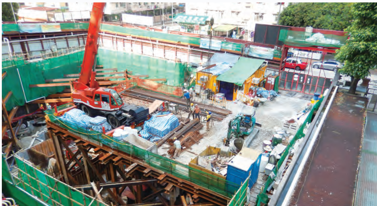
Proposed residential development at No. 11 Grampian Road, Kowloon 九龍嘉林邊道11號建議住宅發展項目
