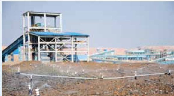
Spray leaching operations in the No.1 stockpile of heap leaching system of Muliashi
