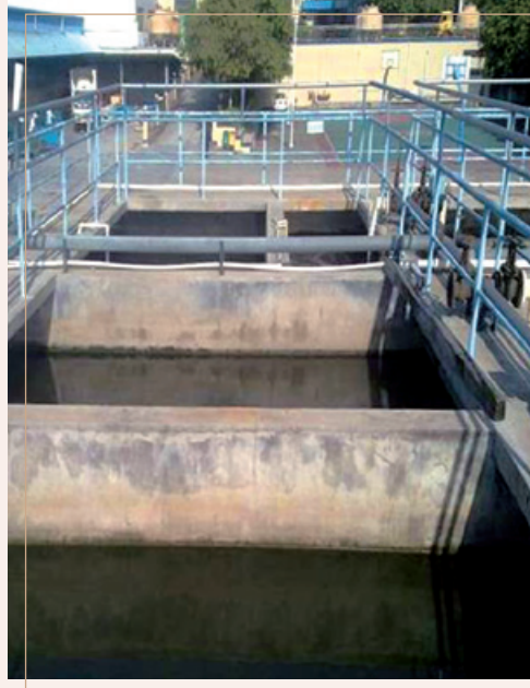
Sanitary water treatment facility
