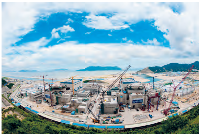
The full picture of the construction site of units 1 and 2 of Taishan Nuclear
