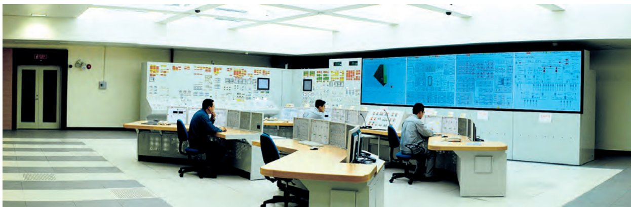
The full-scope simulator training site at Lingdong Nuclear Power Station.
