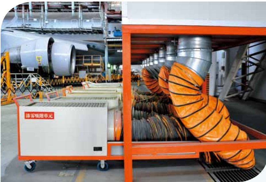
Aircraft Painting Extraction System Inlet and Exhaust at HAECO Xiamen
