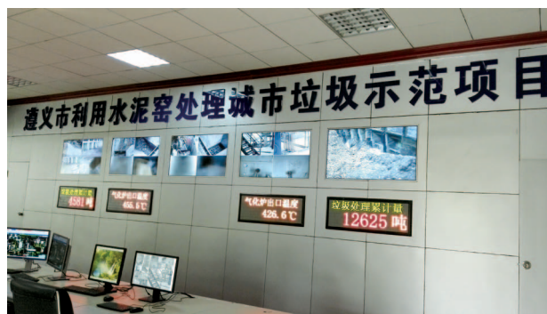
The project regarding cement kiln co-processing of household garbage in Zunyi, Guizhou Province were completed and put into operation in December 2014
