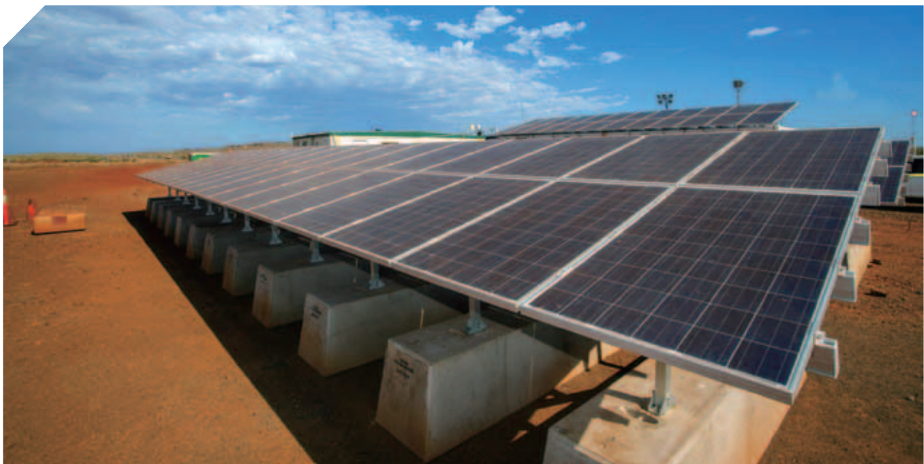
A solar photovoltaic array at the Balmoral gatehouse
