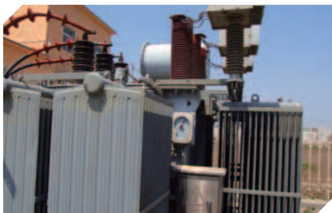
Yuedong Oilfield: Power compensation device
