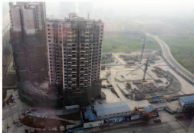
■ Three residential towers in the first stage of the composite development in Chengdu - superstructure works in progress
