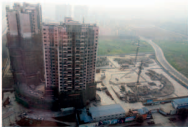
■ Three residential towers in the first stage of the composite development - superstructure works in progress
