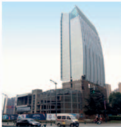
■ Regal Xindu Hotel, a five-star hotel in the first stage of the composite development - superstructure works in progress
