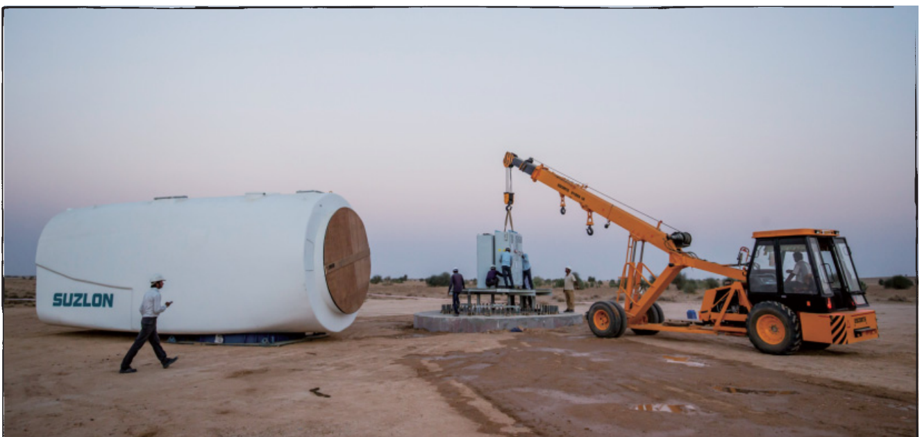
CLP continues to expand its renewable energy portfolio and maintains its position as India's largest wind power developer
