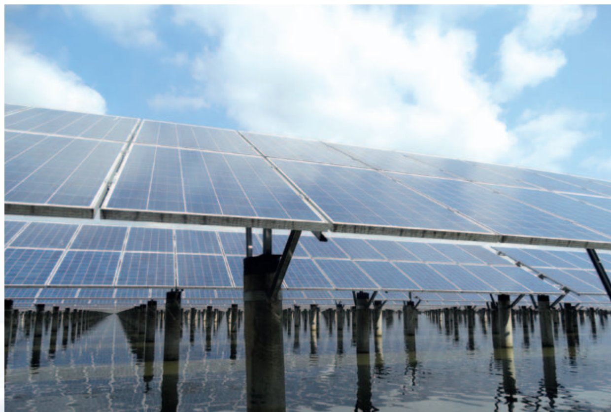
100MW-fishery-photovoltaic power project at Jinhu, Jiangsu
