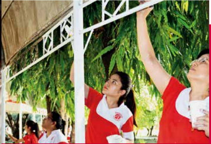
In the Philippines, where as a result of torrential rains and high humidity many public schools require constant maintenance, AIA made possible the repainting of a Maths building at a local school. Over 80 classrooms have been donated across the country since 2011.
