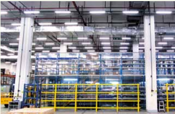
Newly installed LED lights in a storage room at HAECO Xiamen.
