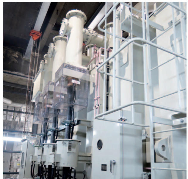
Replacement of the Admiralty substation transformer will improve safety and reliability.
