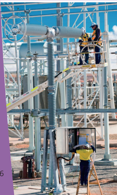
SAPN's Oxiana substation connects the Prominent Hill gold and copper mine to the grid.
