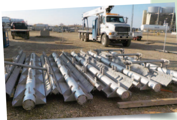
Duct burner equipment being staged prior to installation at a Canadian Power facility.
