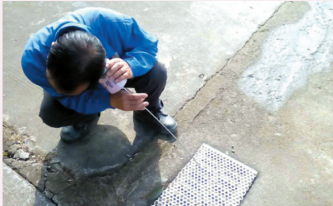
Using leak detectors to locate unseen leaks
