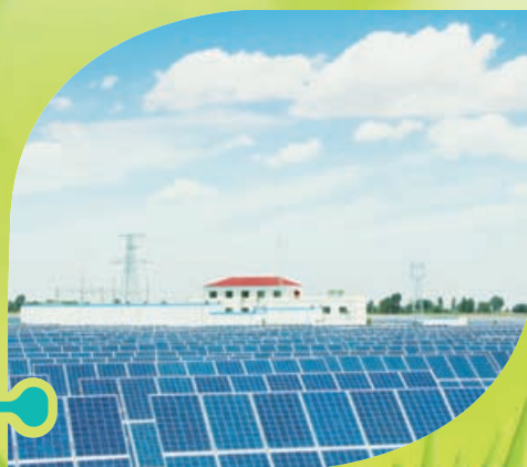
Gansu Wuwei Photovoltaic Power Project
