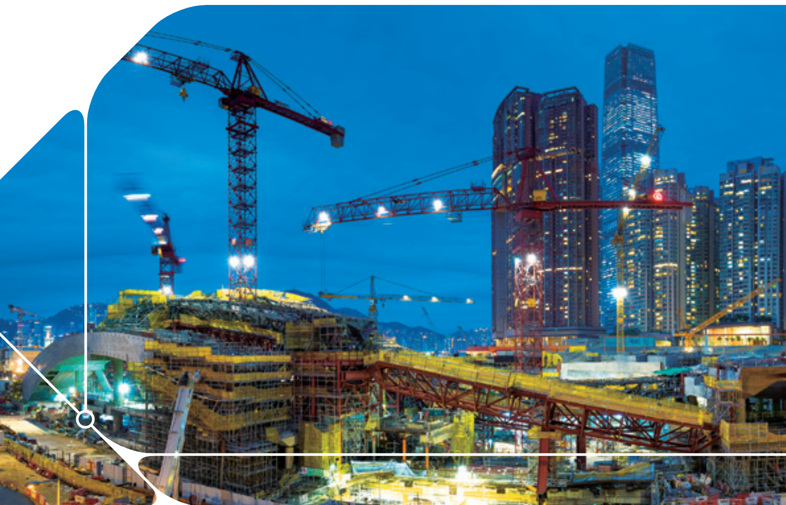
The Express Rail Link will connect Hong Kong to the Mainland of China's high speed rail network
