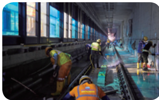
The completion of track laying works was one of the major milestones achieved for Kwun Tong Line Extension in 2015
