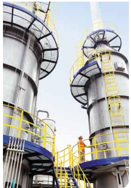
Our coke oven gas plant in Xuzhou, Jiangsu province is expected to undergo operational trials in mid-2016, with an annual output capacity of 110 million cubic metres of LNG.
