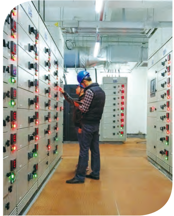
The Group undertook data centre project
