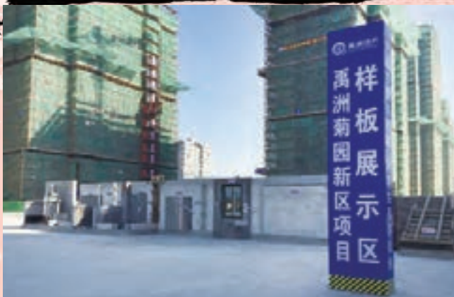
The innovative and excellent management approaches of The "Safe Construction Planning" applied in Yuzhou Bustling Center in Shanghai are promoted in the whole Group 集團推廣上海禹洲·老城里項目的「安全文明施工策劃」等創新、優秀管理方法
