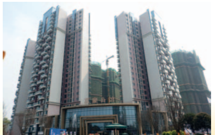
■ Three residential towers in the first stage of the composite development – nearing completion
