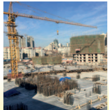
■ Superstructure works of the residential towers of the composite development in progress
