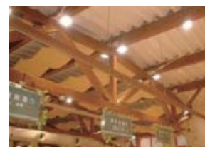
LED lighting within a hall
