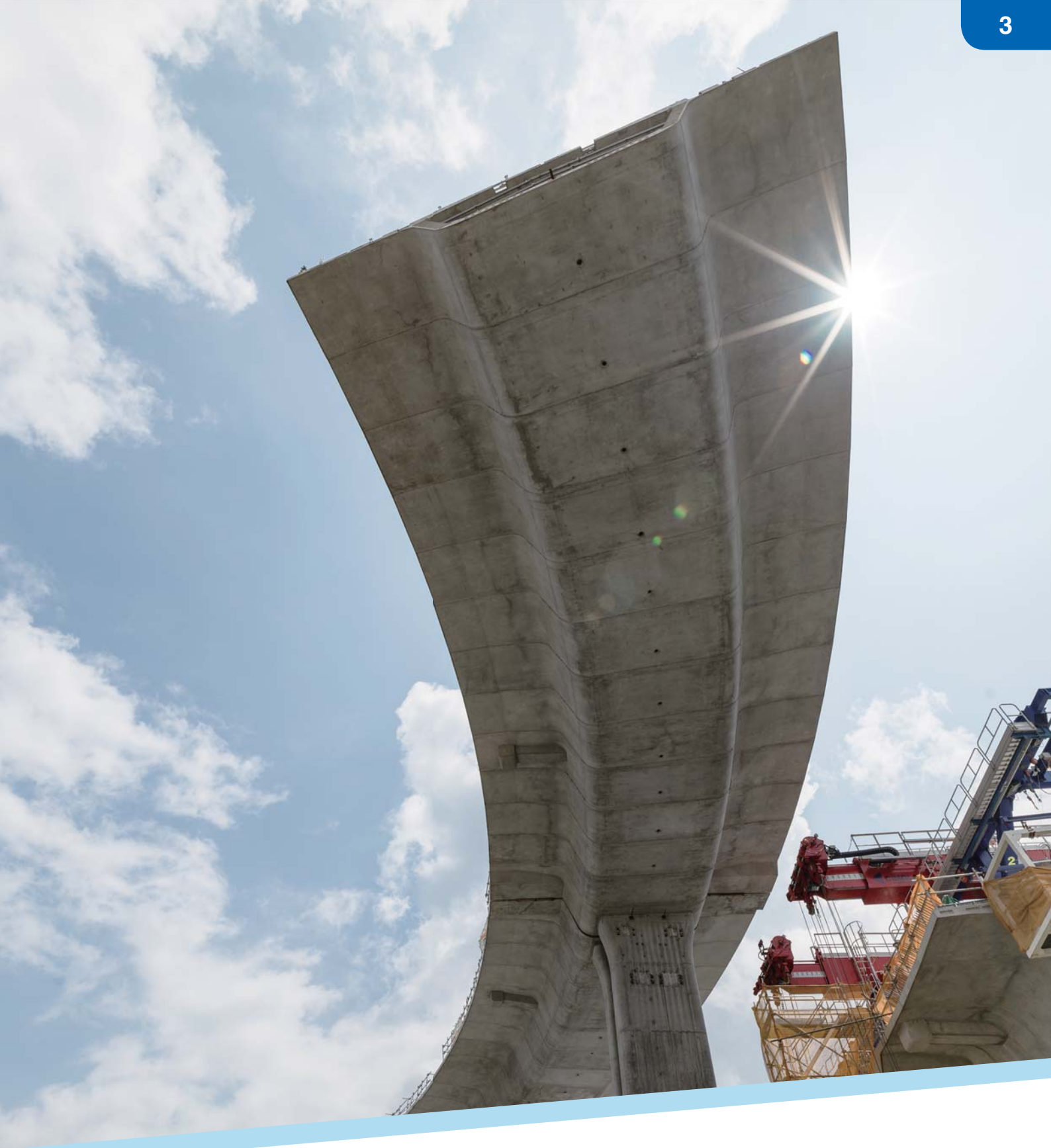
1-3. Liantang/Heung Yuen Wai Boundary Control Point, Site Formation and Infrastructure Works – Contract 3 蓮塘／香園圍口岸土地平整及基礎建設工程 — 工程合約三
