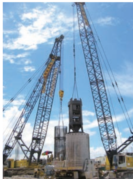
Bored piling work at a construction site undertaken by Kin Wing Foundations Limited
