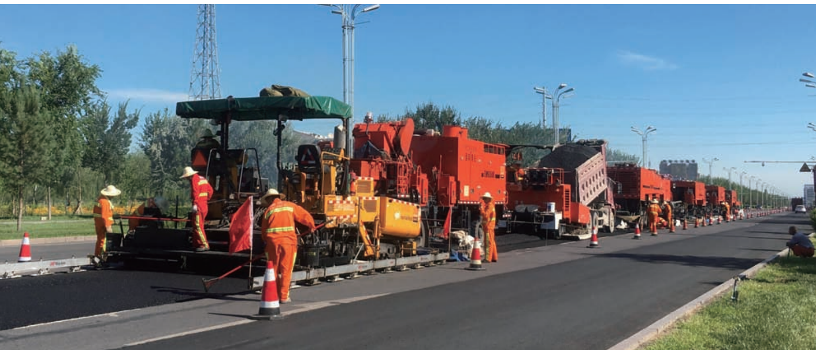
APM Service Project in Xinjian, PRC
