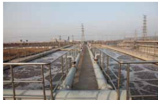
Changmao Lianyungang – Waste water processing system
