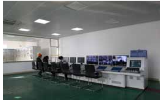
Changmao Lianyungang – Control room of maleic anhydride production line with annual capacity of 10,000 tonnes using butane production method
