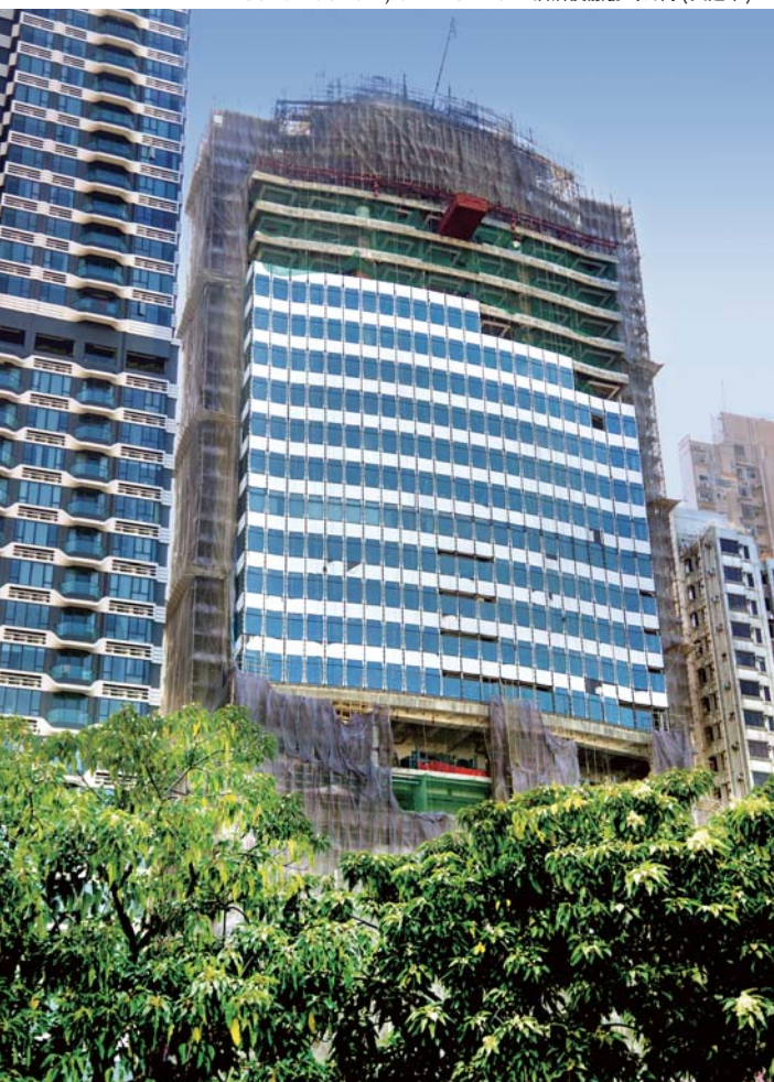
ONE-EIGHT-ONE HOTEL & SERVICED RESIDENCES ( UNDER CONSTRUCTION ) ONE-EIGHT-ONE酒店及服務式公寓 (興建中)
