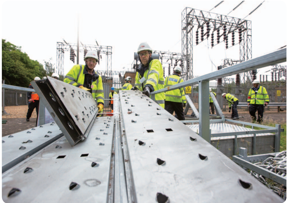
UKPN staff in action at a network site to maintain reliability standards.
