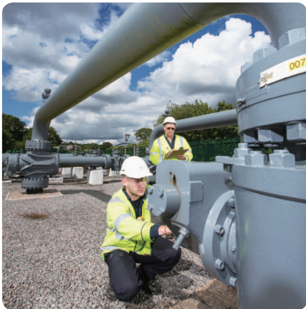
WWU staff carry out checks on network equipment.
