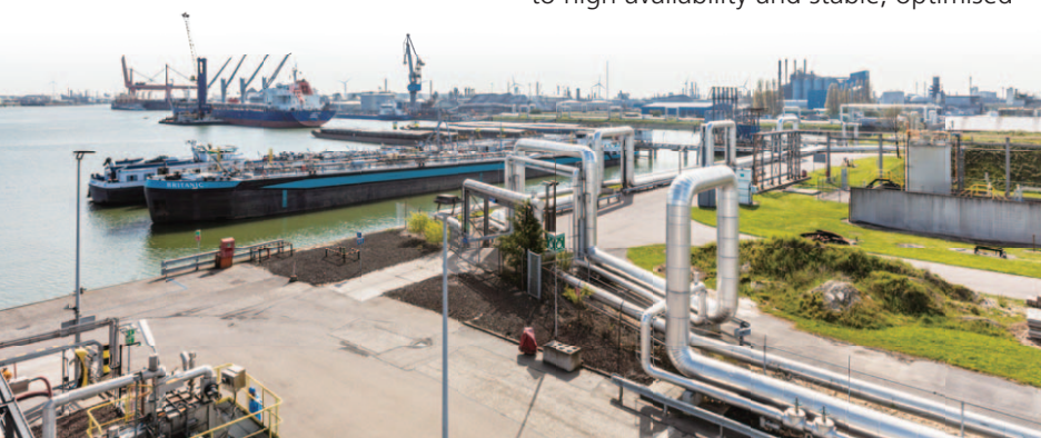
AVR network pipes deliver steam to customers in Rotterdam Port.
