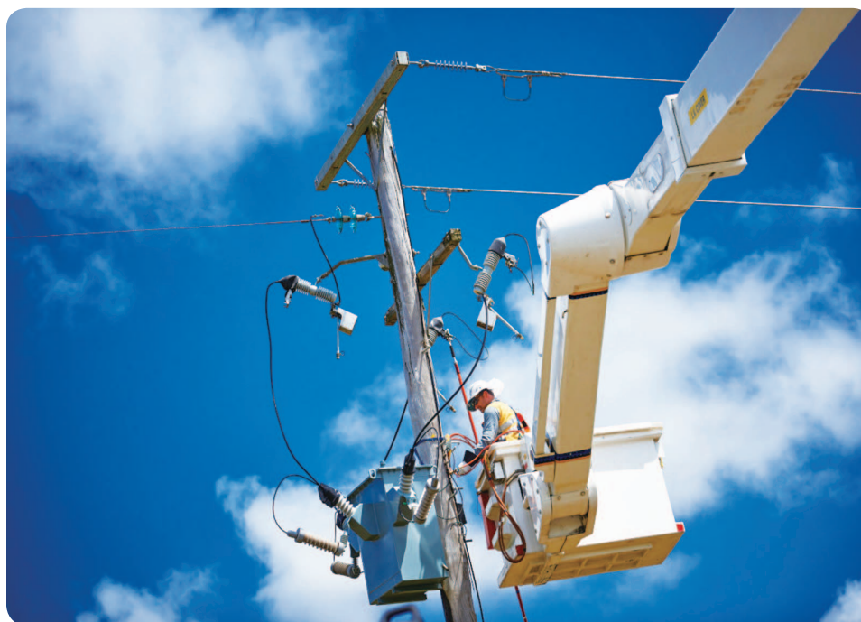
New high-voltage lines installed on the Powercor Network near Mildura in north-western Victoria.
