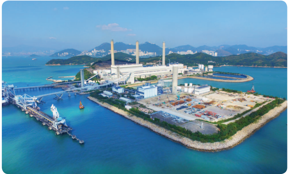
Construction of new gas-fired units in progress at HK Electric's Lamma Power Station.
