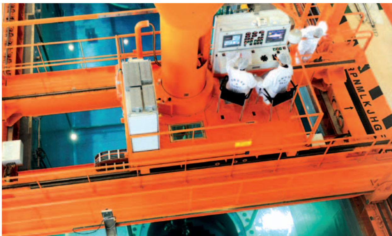
Outage personnel carried out the refueling work during the unit outage period
