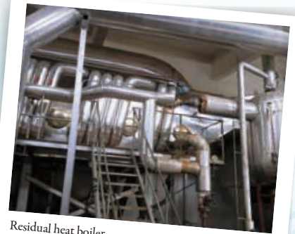
Residual heat boiler
